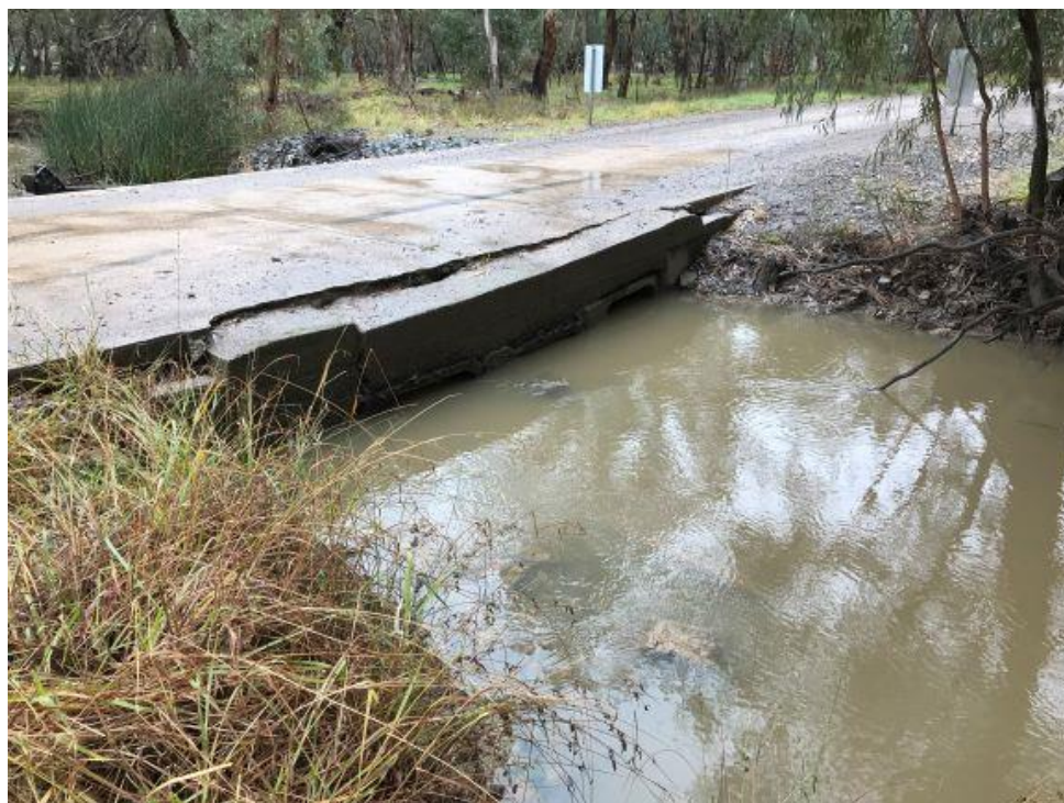
Figure 28: The culvert under Kokoda Road (reach 1 of lower Broken Creek) is expected to be a barrier to fish passage
